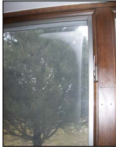
Broken seal between glass.
