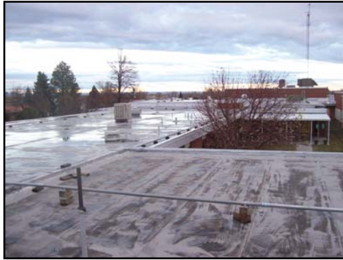
View from area 'D', ponding on area 'C'.
