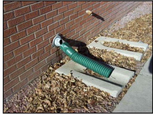
Downspout draining near the building.
