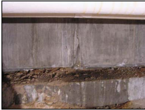
Crack in the foundation with moisture seeping through.
